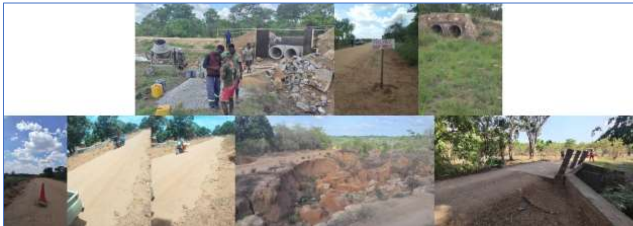
Figure 11: Observed Road Conditions
